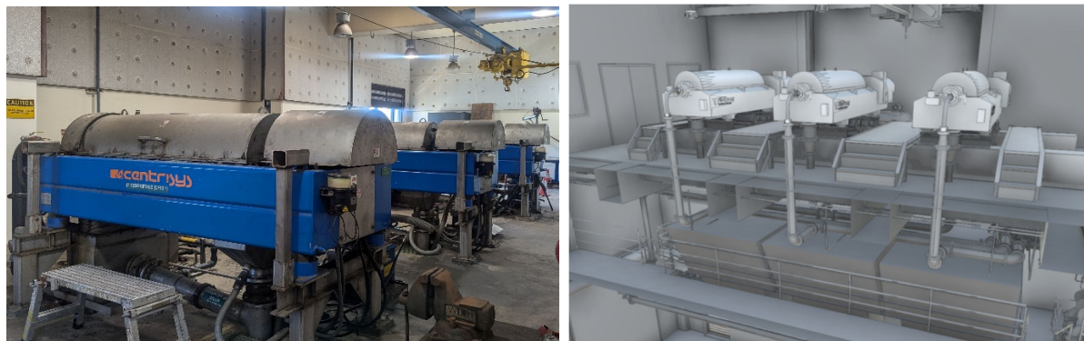
Existing Centrifuges (left) and 3D Model of the centrifuge room with the new centrifuges (right)
