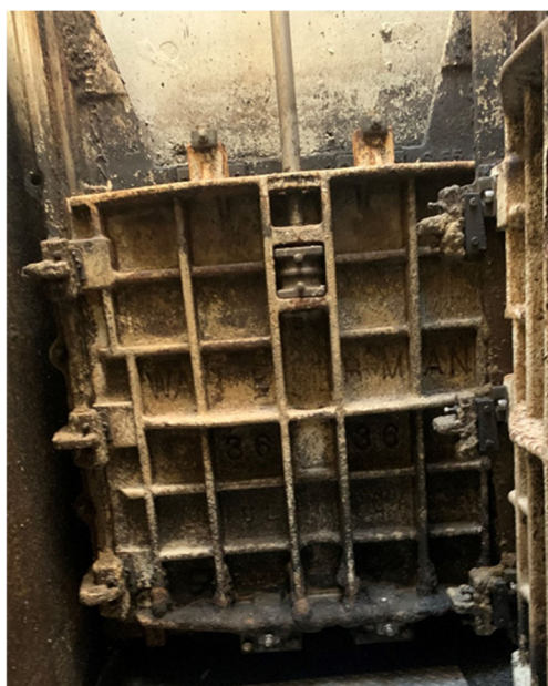
Originally installed cast iron sluice gate
