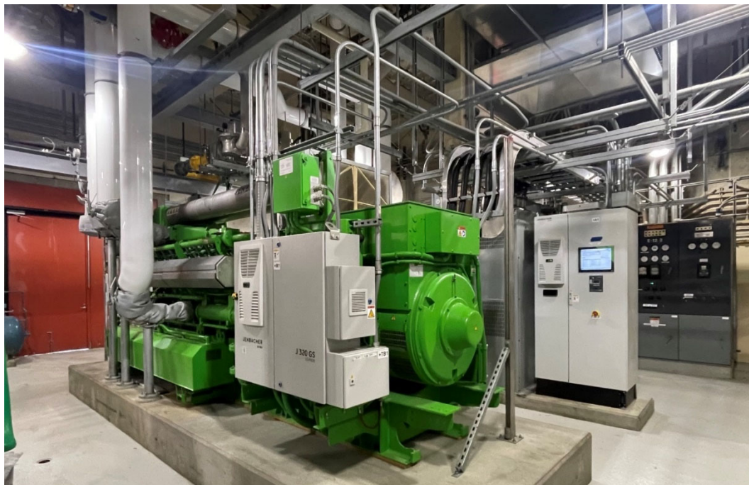
New cogeneration engine
