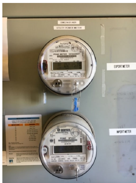
Power export meter to track energy being sold to MCE.
